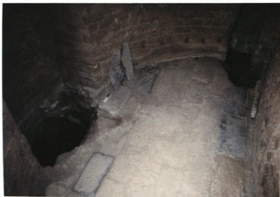
Fig. 12. Toilet room of the External Nymphaeum at the Water Court (31) with collection box (left), down spout for rainwater (right) and gray slates as floor decoration (photo R. Kragting).
