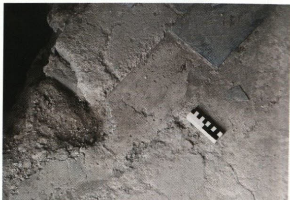
Fig. 13. Detail of the toilet floor in the External Nymphaeum at the Water Court (31) with lead water pipe ending in collection box (top left) and small pipe next to metre-stick (photo R. Kragting).
